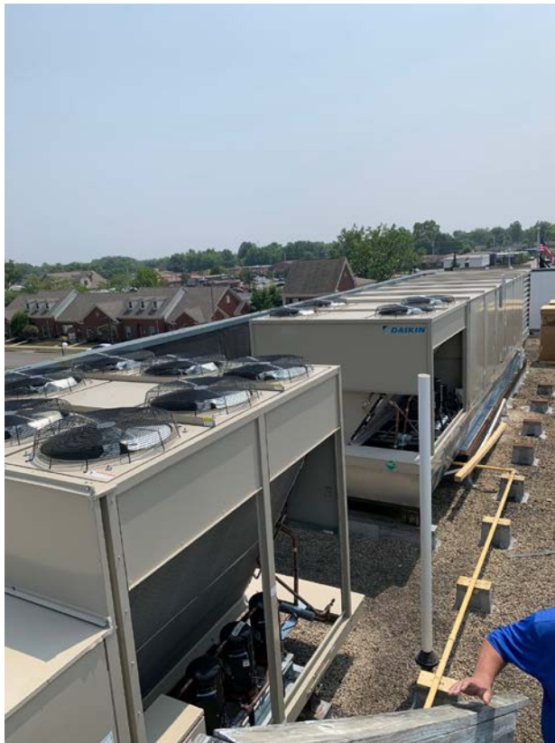
Justice Center RTU's
