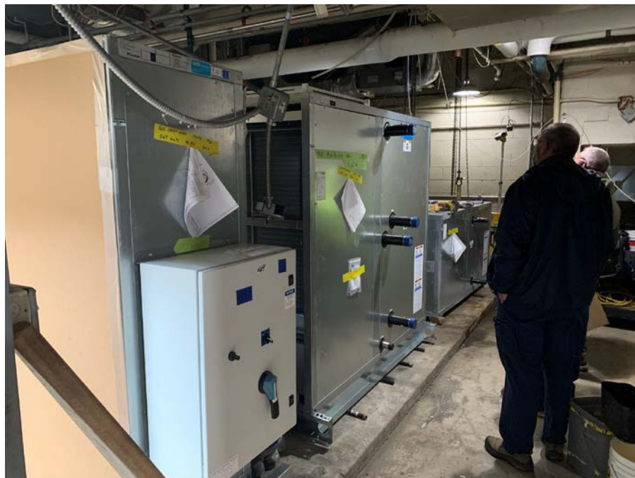
Air Handling Unit
